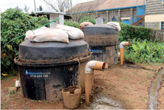
Biodigesters. Source: Takamoto Biogas
